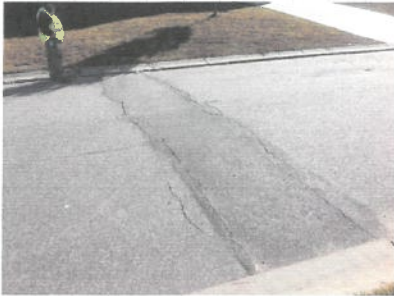
30 ft curb damage in front of house 333 Blythe Creek drive. An additional 30ft curb damage across street Also a utility crossing road failure of 12x24
