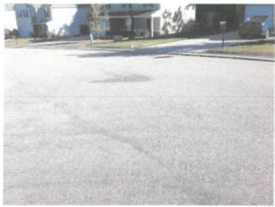
60x24 longitudinal cracking and reflective at intersection of broken arrow ct and Blythe creek dr
