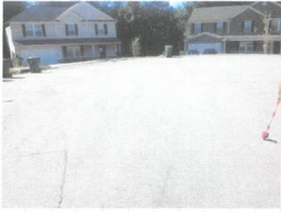
Cul de sac 96x80 alligator and reflective cracking. 87 ft curb damaged binder course surface course not installed
